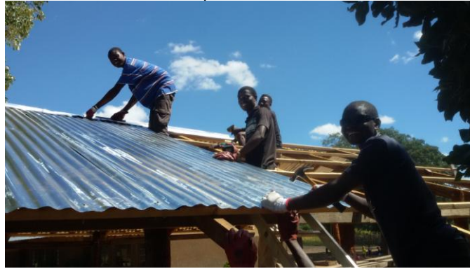
Below: Cholwe, Zulu and Kelvin busy with the roof to our new preschool.
